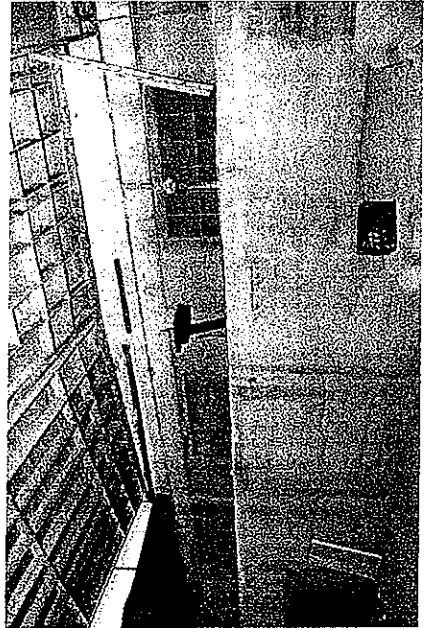
Int balcony N end #21 Interior. First walked to north end of building. Interior balcony for storage and stacking.
